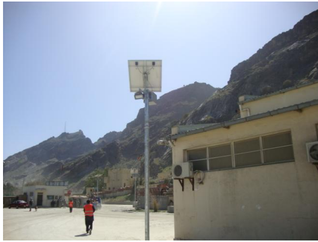
NST Floodlight At Middle East US Army Base
